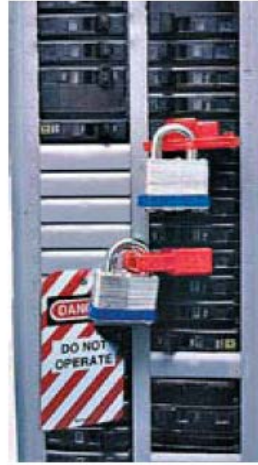
Danger tagged circuit breaker locking off devices
