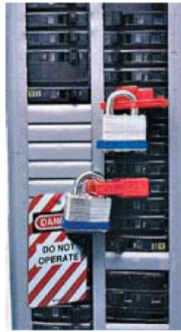
Danger tagged circuit breaker locking off devices
