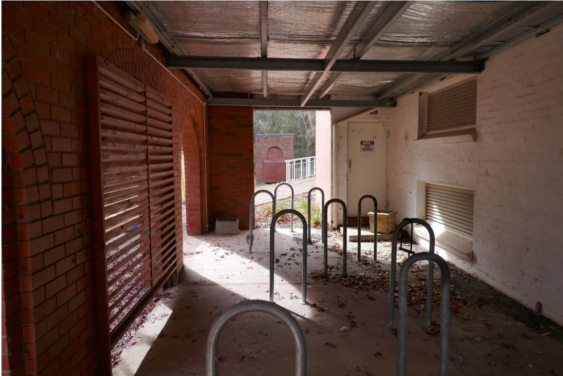
Figure 31 Dugout: view looking north, with the original west elevation at right, and the 1980s screen wall at left
