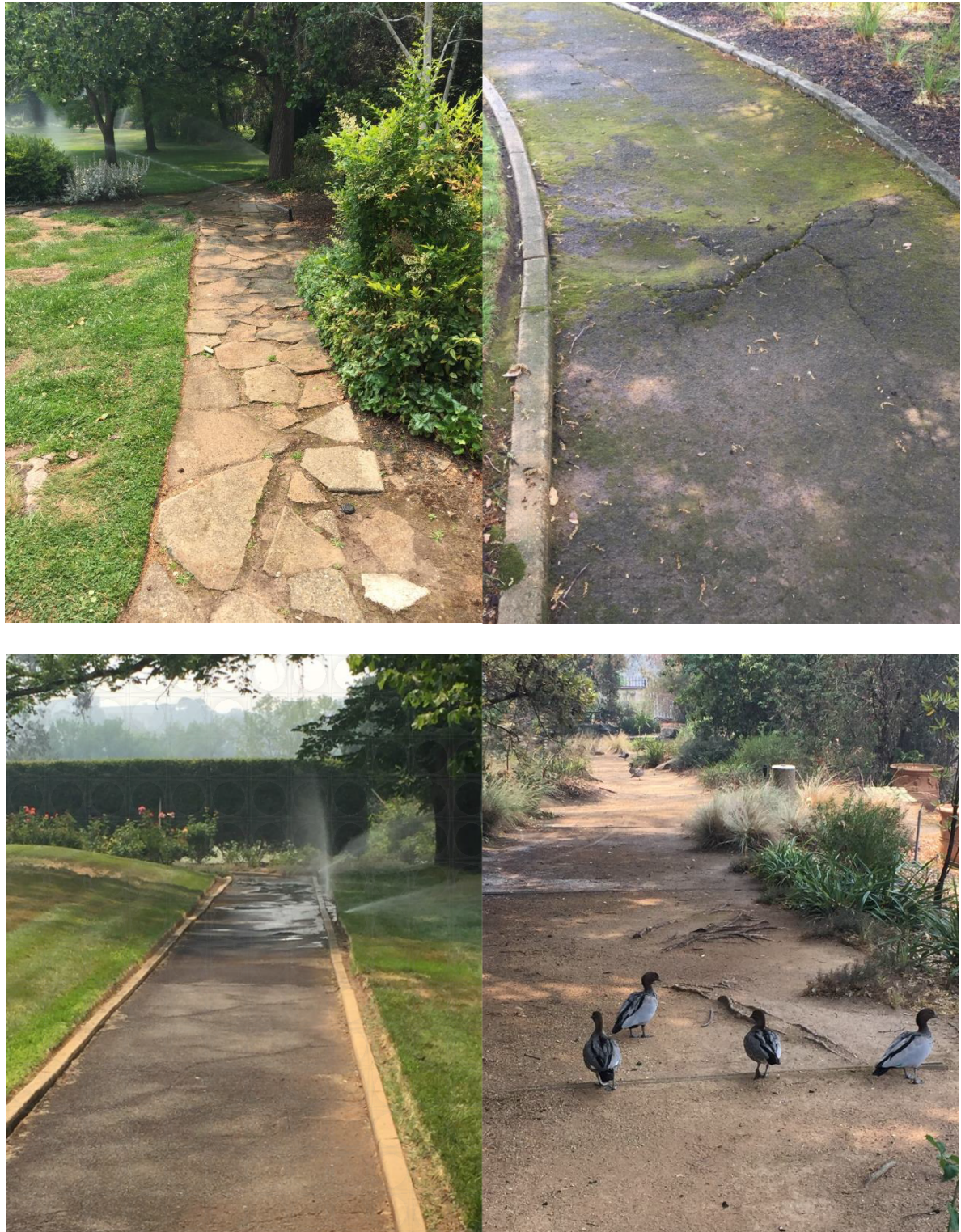
Figure 19: Examples of Potentially Hazardous Paving (most of which was remediated in March 2023)
